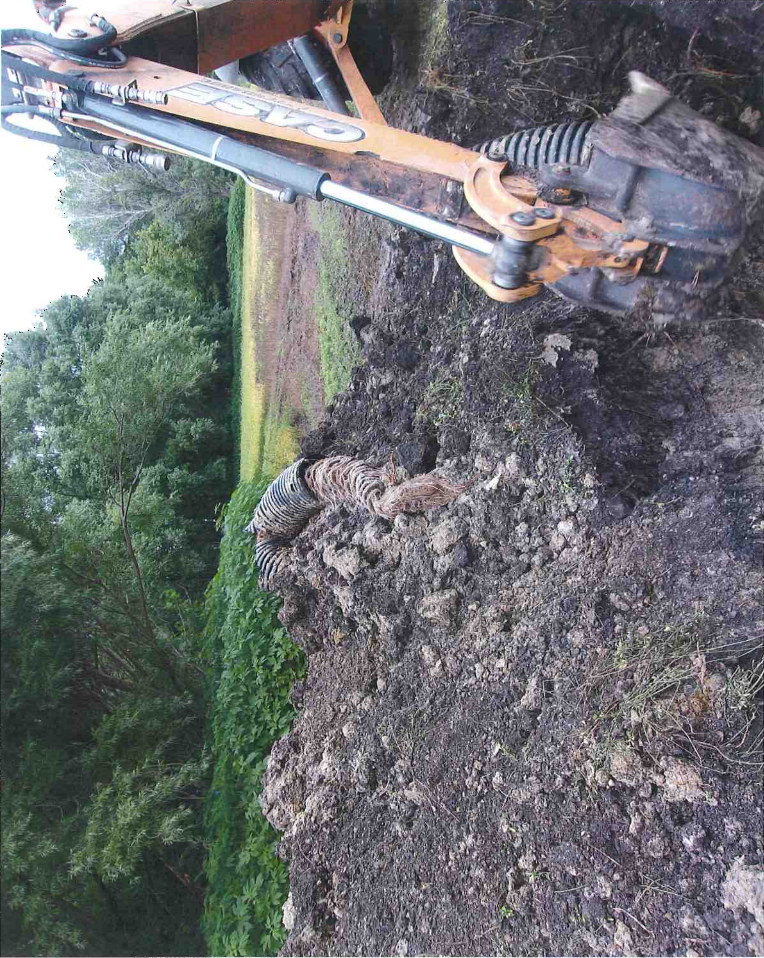
TILE TOTALLY RUINED BY ROOTS, HAD TO REMOVE
