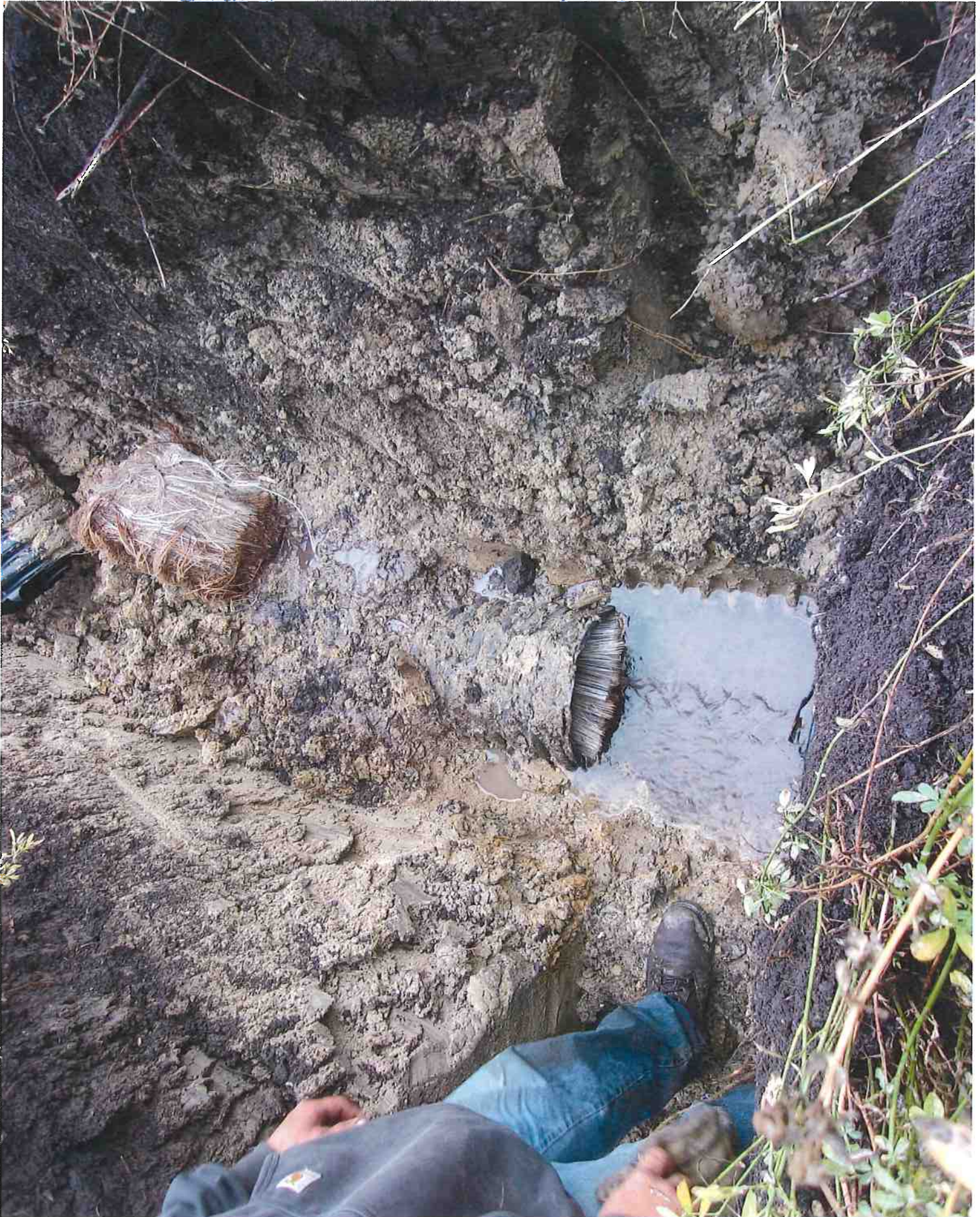
SECTION OF 12" PLASTIC TILE REMOVED EXPOSING TREE ROOTS
