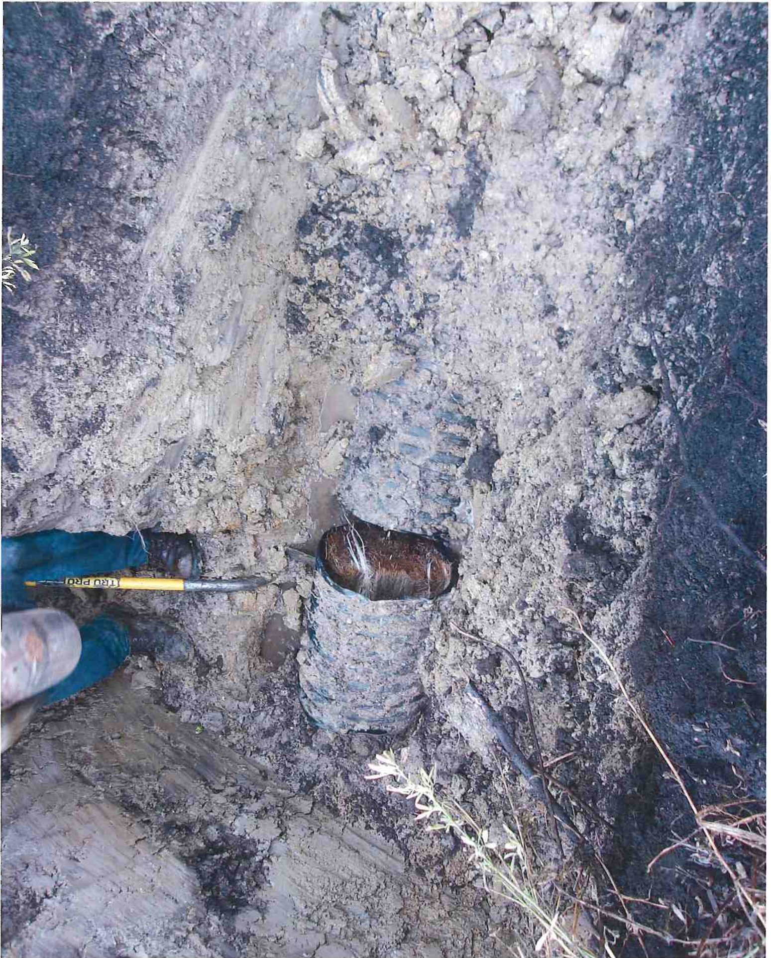
TREE ROOTS IN PLUGGED 12" PLASTIC TUBE
