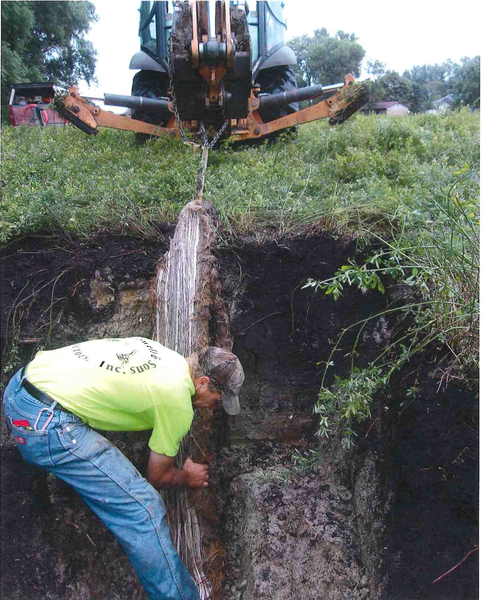
Roots Pulled From TOTALLY PLUGGED 12" TUBE
